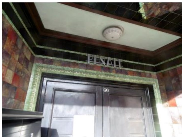
Entry doors and tiles
